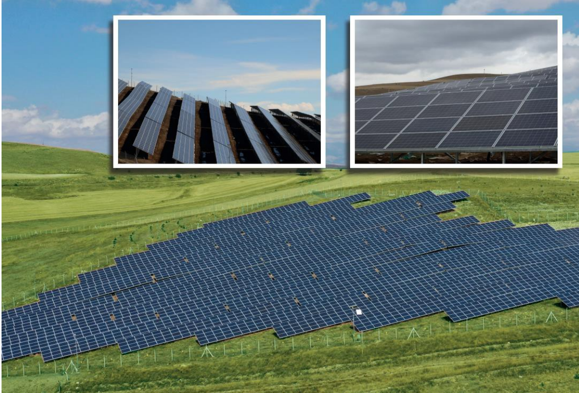
Baberti Campus Solar Power Plant
