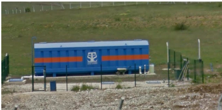
Domestic Package Wastewater Treatment Plant
